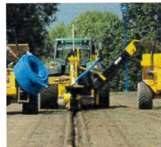
Alternatively, the drainage trenches can be cut straight through the turf. The drains are installed, and then
